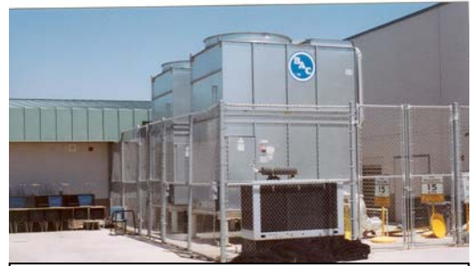
Typical MiniBrom Treated HVAC Cooling Tower
