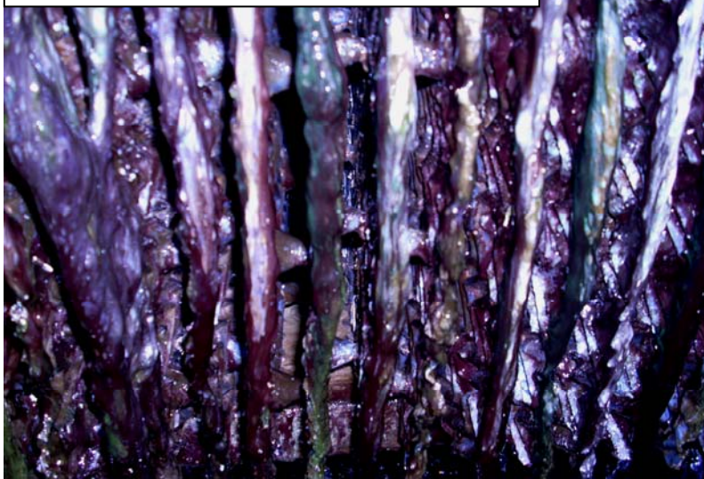
Algae Growth - Cooling Tower Fill
