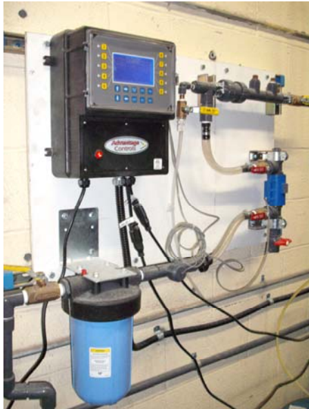
Installed BlueTrak Control
