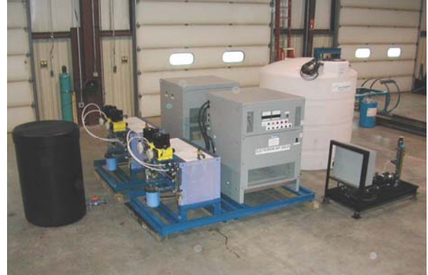
Two EB-60 units with dose tank and pump.
